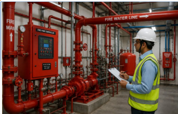
Fire Protection Systems
